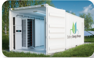
Power Conversion Systems
